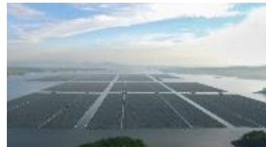
Cirata Floating Power Plant, Largest Floating PP in Indonesia (2021)
